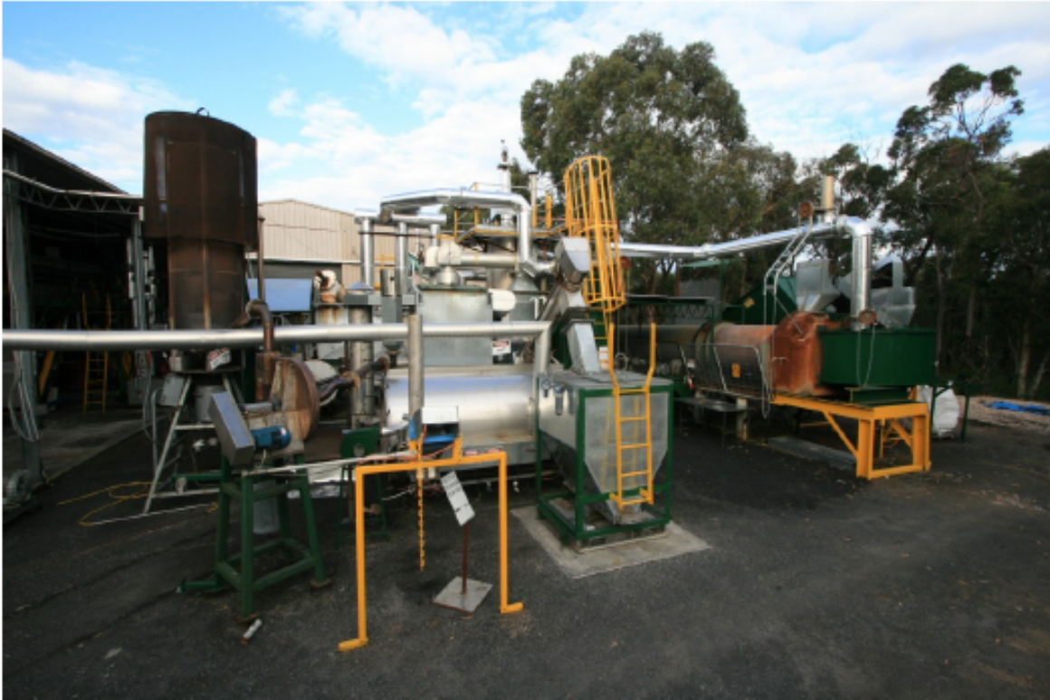
Figure 6: BEST Energies Australia Slow pyrolysis plant. (Pacific Pyrolysis, 2011).
